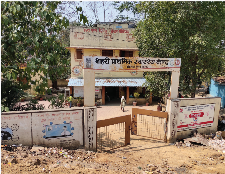
The level of the health facility from the road level makes it vulnerable for water flooding in during heavy rains
